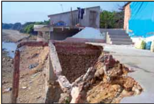
Damage caused to housing by flash flooding
