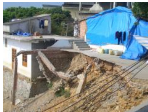
Damage caused by Hurricane Damrey
